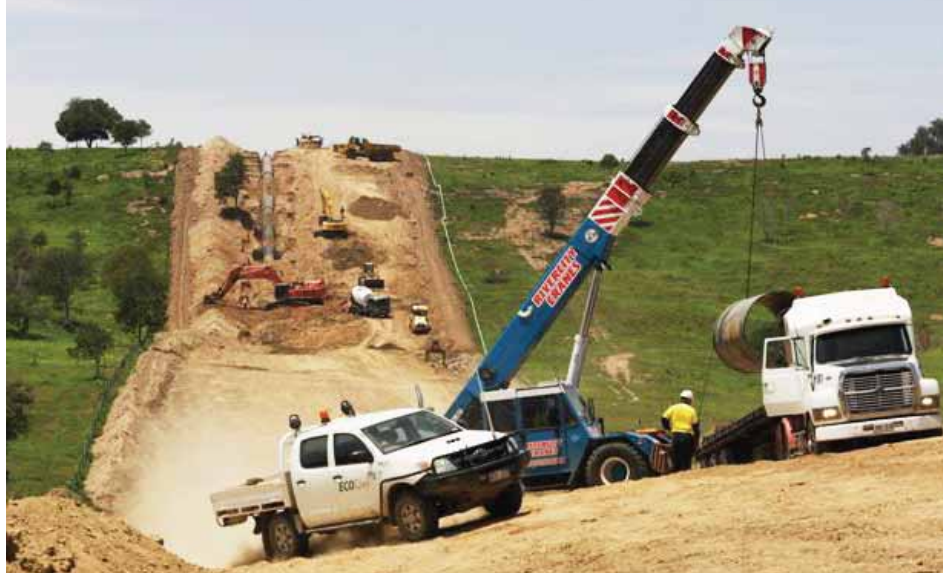
Western Pipeline Alliance laying large-diameter pipeline up one of the hills on the way from Bundamba to Tarong Power Station
